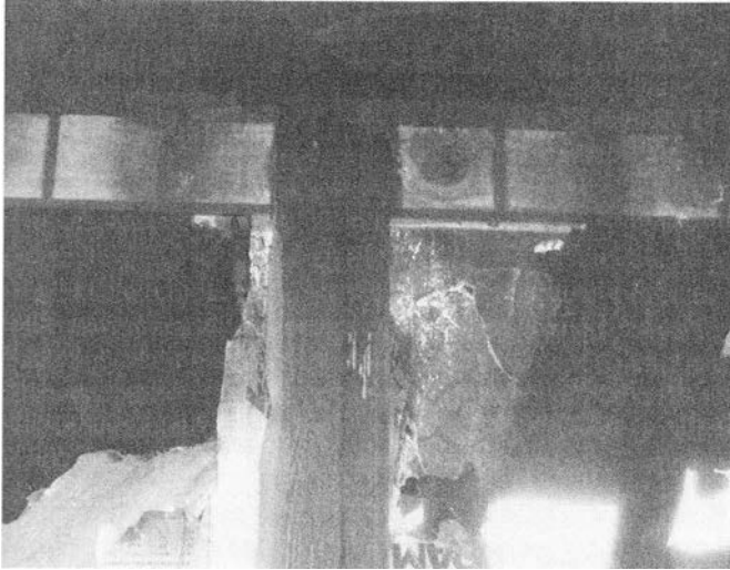
Figure 6.4 Fire-damaged timber floor beam
