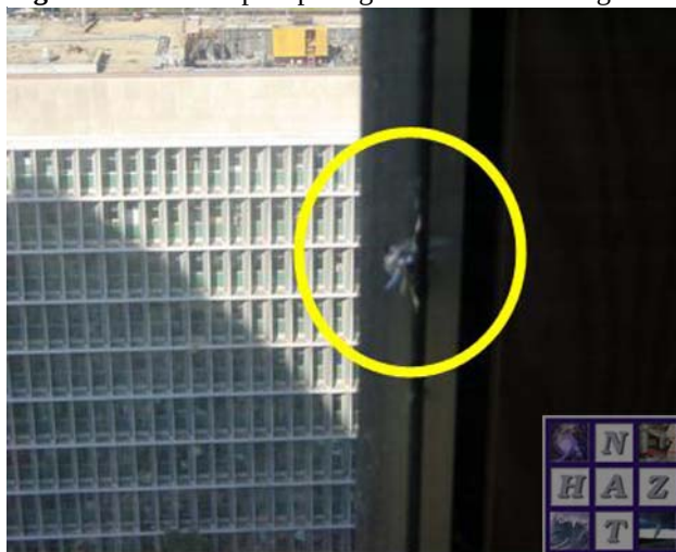
Figure 8 Missile impact pitting on Amoco Building.
